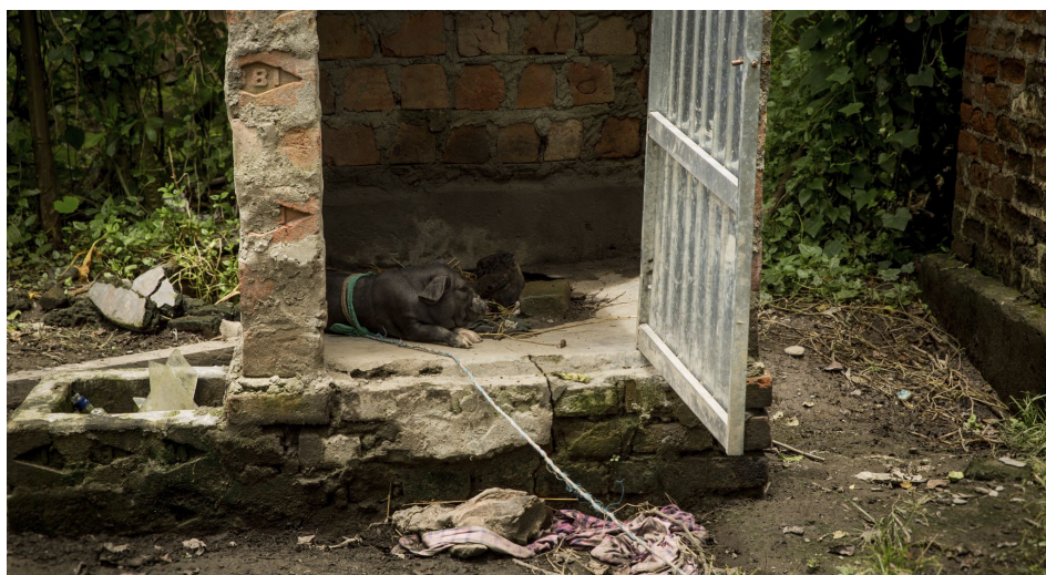
The state of a toilet provided for workers. Photo: Roanna Rahman/Oxfam
